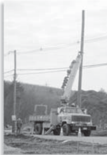
GELD AT WORK Our linemen installing one of the new riser poles where the underground service from the Route 119 widening project will join with the current overhead lines.
